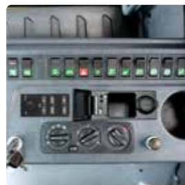
Centralized Instrument Switch Panel
